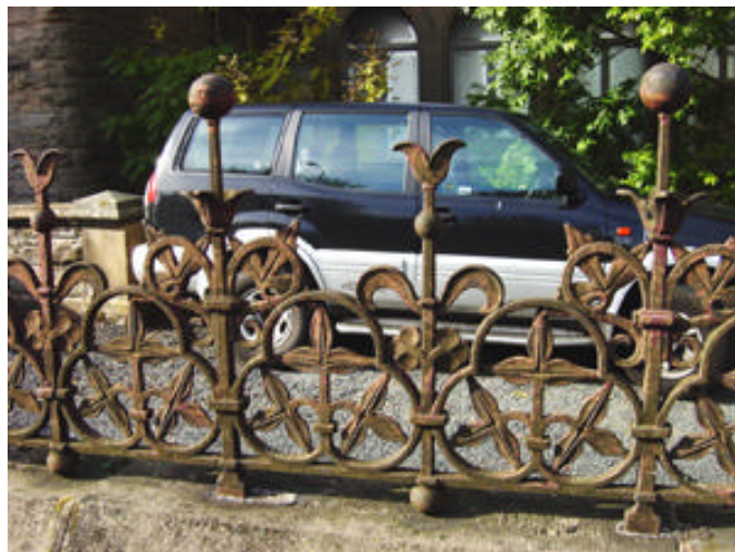
Railings installed in the 1920's to replace originals. Note pitch has been altered
