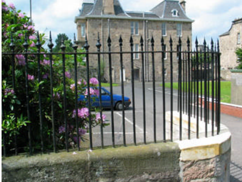
Original cast iron railings with mild steel railings installed to the right.
